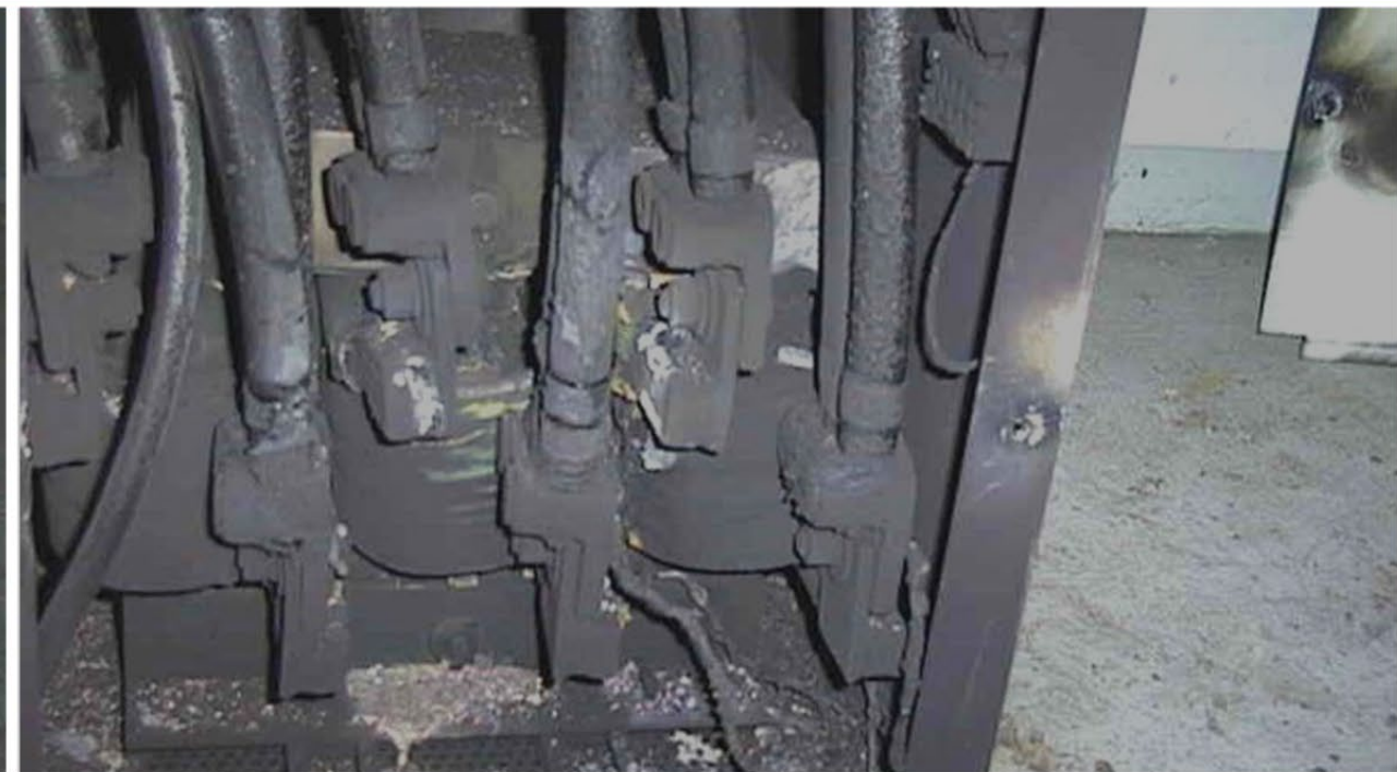
EXAMPLE ENCLOSED TRANSFORMER
